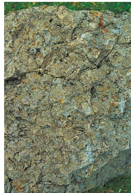
Poor Condition VS = 0
